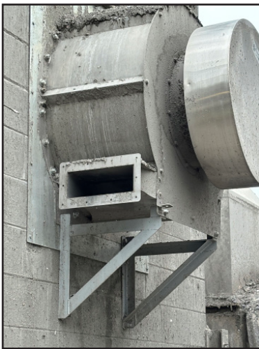
ACB T-50 unit installed at a Recycling Plant.
