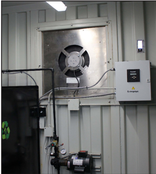
View of the same ACB mounted to the wall from the clean-air side.
