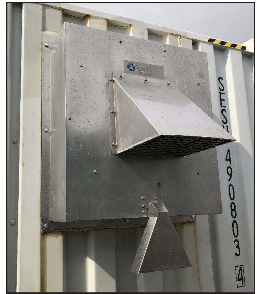
Outside view of an ACB unit mounted to the wall at a mine.
